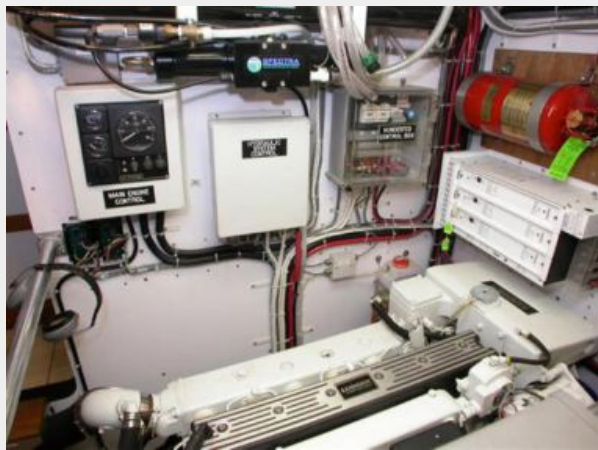
Engine Room detail 1
