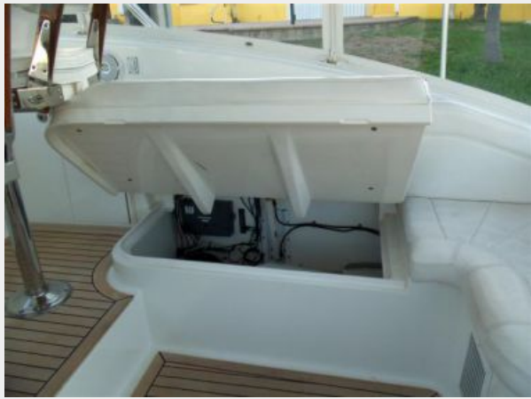
Hydraulic Storage Hatch
