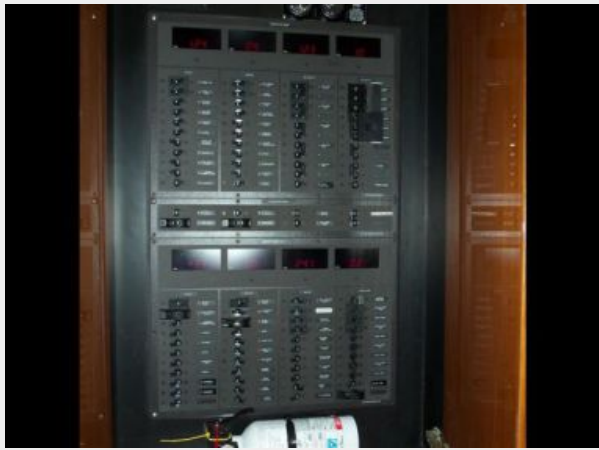
Salon Electrical Panel
