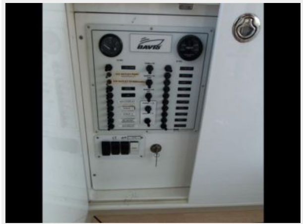
Cockpit Breaker Panel
