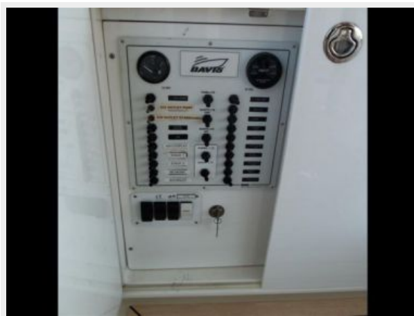
Cockpit Breaker Panel
