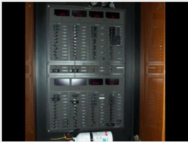
Salon Electrical Panel
