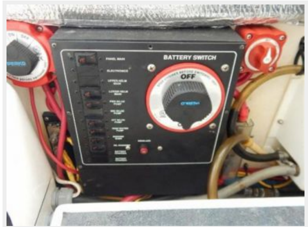
Engine Battery switches
