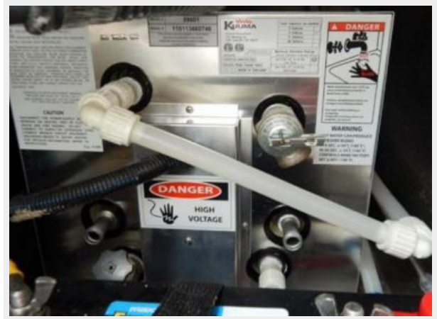
New Hot water heater
