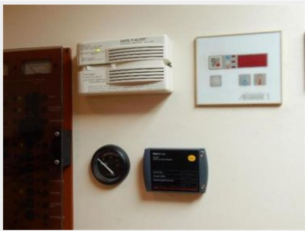
Salon Control Panels Close up
