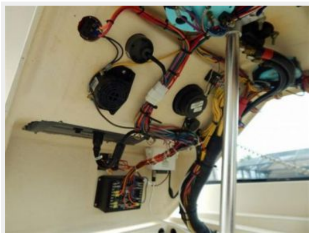
Cockpit Helm Wiring
