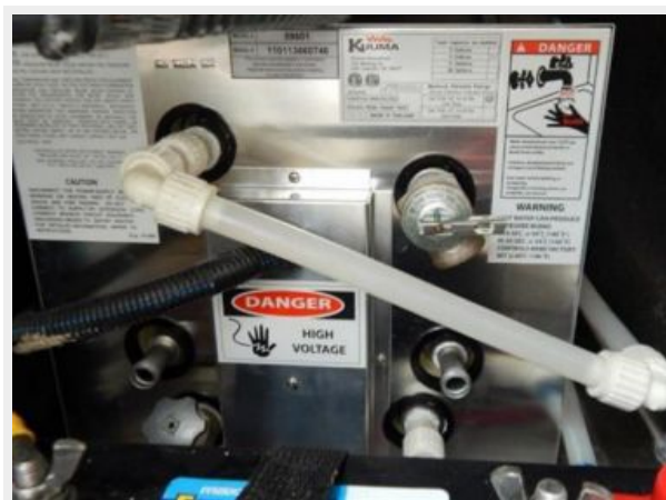
New Hot water heater
