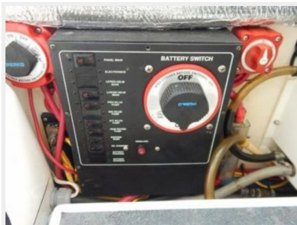
Engine Battery switches
