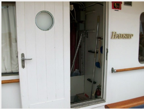
Engine room entry
