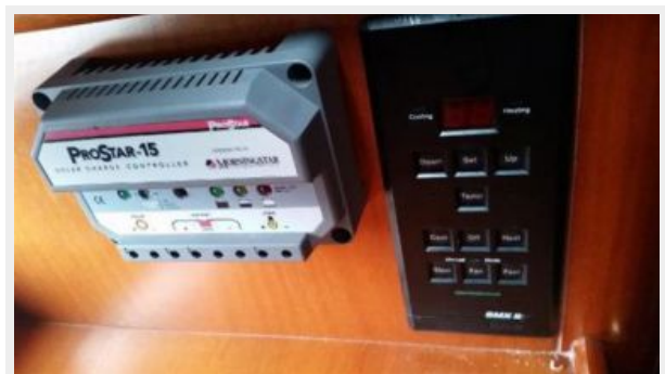
Solar Panel Monitor / AC Control
