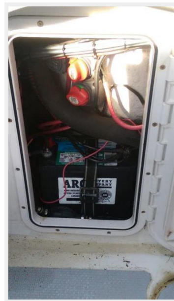
Battery & Switch - Starboard Side
