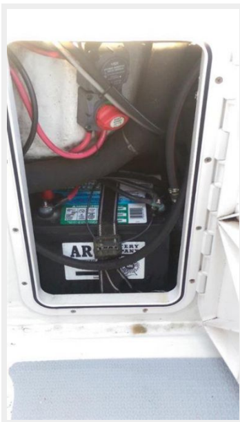
Battery & Switch - Port Side
