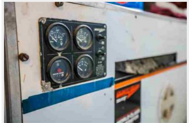
Engine room - 20 kw Northern Lights GenSet
