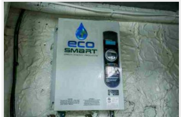
Engine room - eco smart hot water heater
