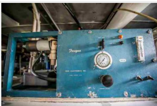
Engine room - water maker
