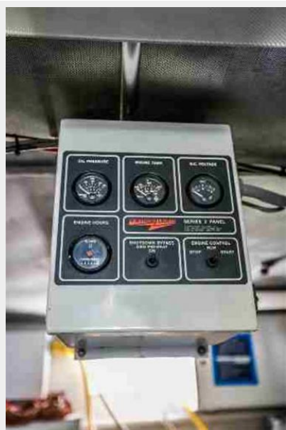
Engine Room - 30kw Northern Lights GenSet
