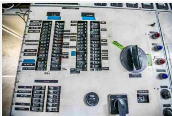
Engine room - control panel
