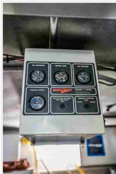
Engine Room - 30kw Northern Lights GenSet
