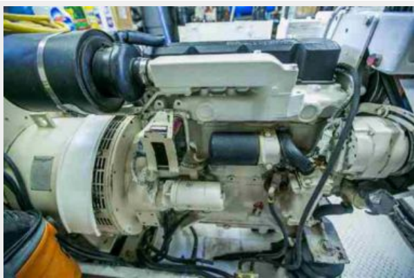
Engine room - 30kw Northern Lights GenSet
