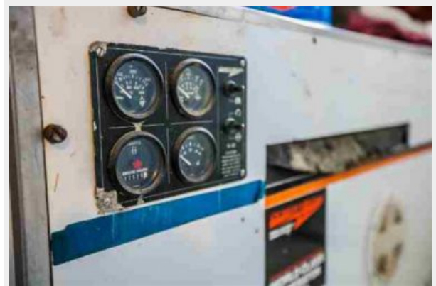
Engine room - 20 kw Northern Lights GenSet
