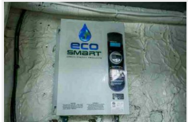
Engine room - eco smart hot water heater
