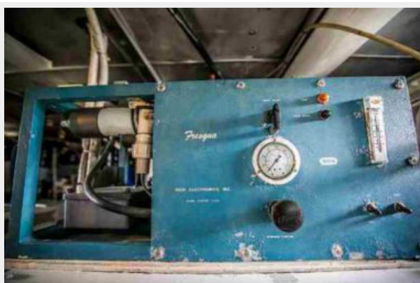
Engine room - water maker
