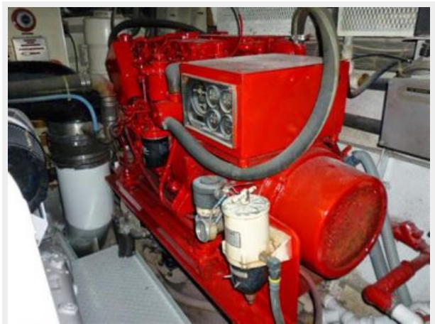
Generator in Engine Room
