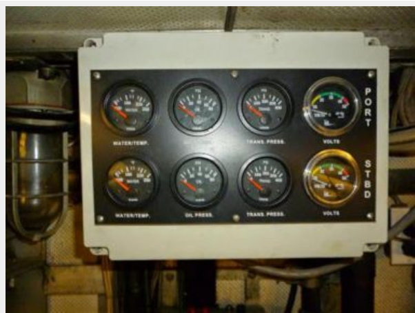
Engine Room - Manual Gauges
