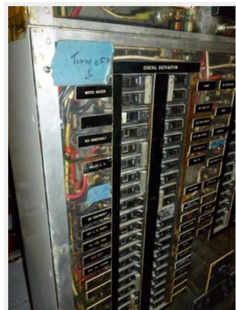
Engine Room - Electrical Panel
