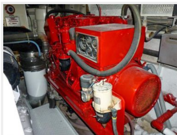
Generator in Engine Room
