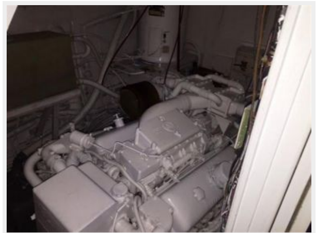
Starboard Engine room
