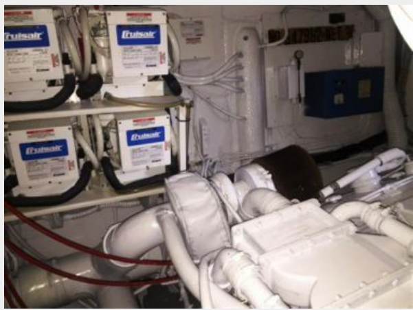
Port engine room
