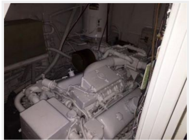
Starboard Engine room
