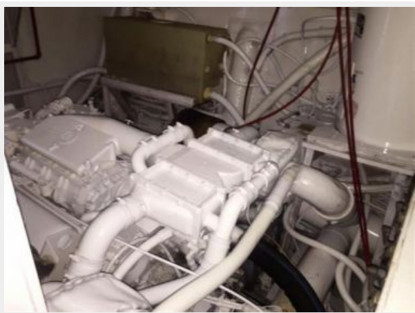
Starboard Engine room
