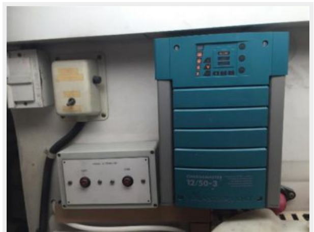
Engine Room - Mastervolt battery chargers 12/50-3
