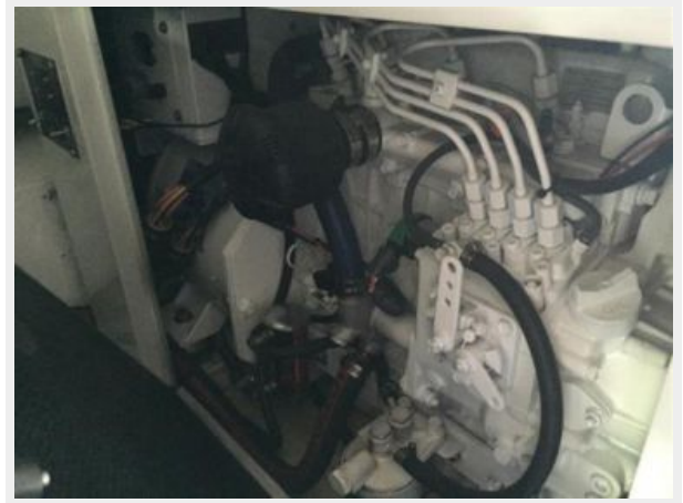
Phasor 12.5kw - Backup Generator
