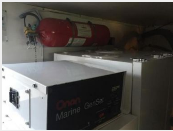
Main Generator - Onan 19kw
