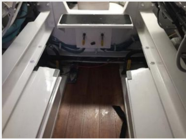
Engine Room - Wood Floor Batteries in fiberglass boxes
