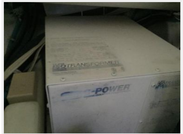
Engine Room - Charles ISO boost/volt stabilizer
