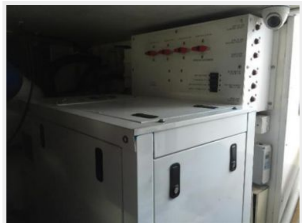
Engine Room - Phasor 12.5kw Backup Generator
