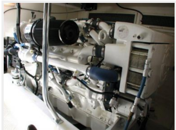
Engine & Mechanical Equipment 2 - Port Engine
