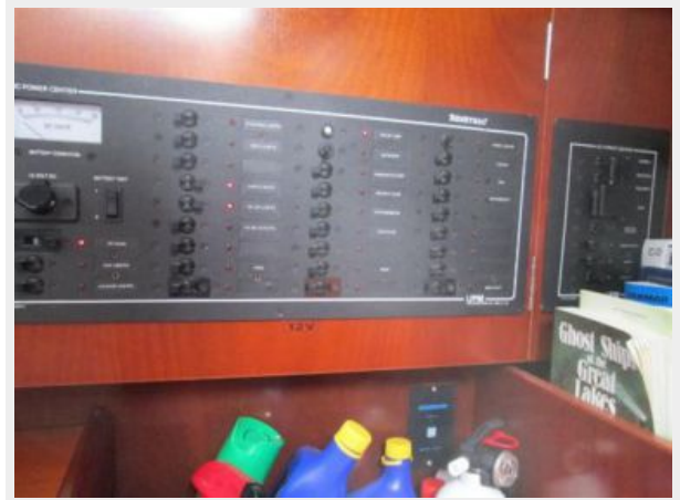
Electric panel at Nav. station to starboard
