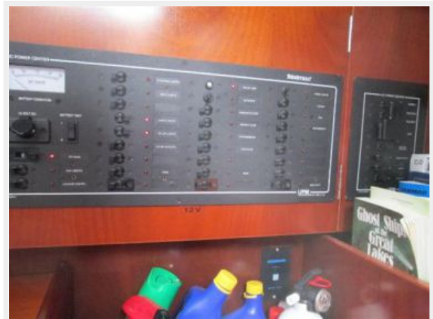
Electric panel at Nav. station to starboard
