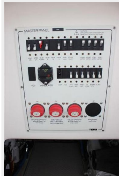
Master Breaker Panel
