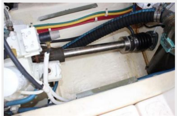
Port drive shaft
