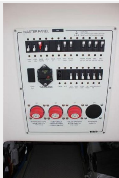
Master Breaker Panel
