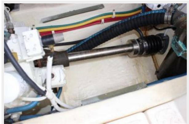
Port drive shaft
