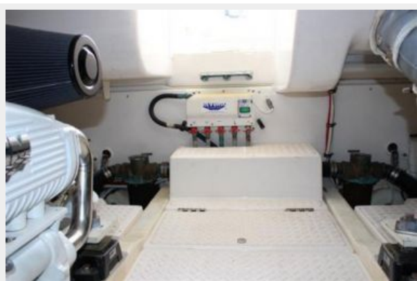
Engine room looking aft
