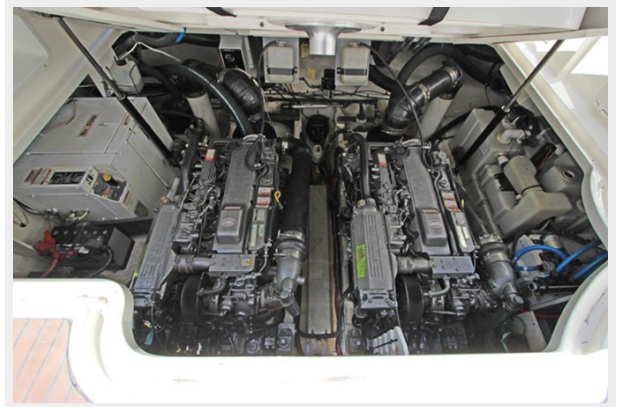
Twin 315 HP Yanmar Diesel Engines & Onan 5kw Diesel Generator In Sound Shield
