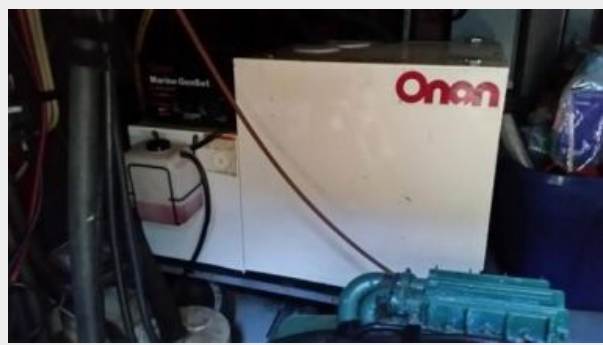
ONAN 9kw Genset (1616 hours)
