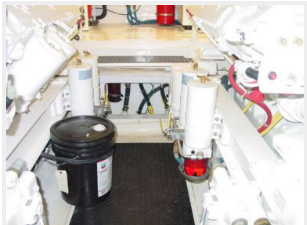
Engine & Mechanical Equipment 8
