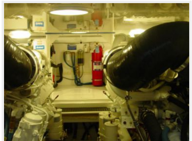
Engine & Mechanical Equipment 2 - Engine Room
