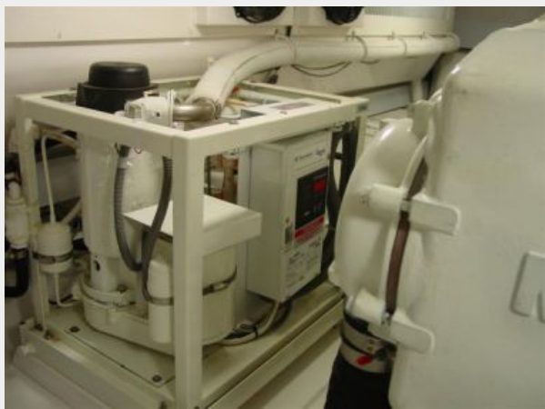
Engine & Mechanical Equipment 5
