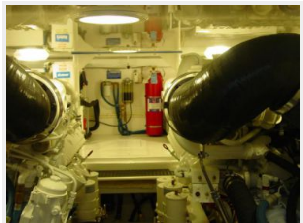
Engine & Mechanical Equipment 2 - Engine Room
