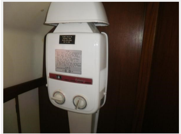
Heater for hot water
