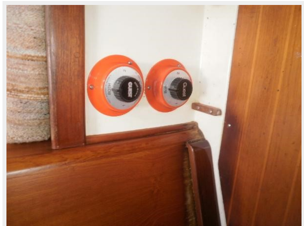
Duel Power Switches w/ Off/ 1/2
