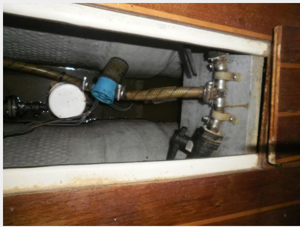
Primary Bilge Pump
