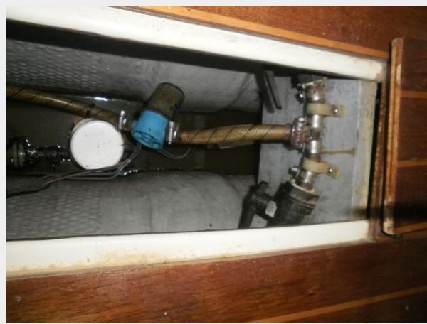
Primary Bilge Pump
