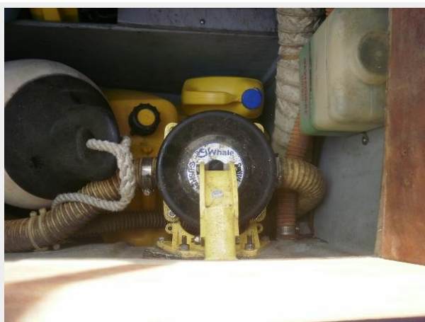
Starboard Aft Storage Locker/Whaler Emergency Pump
