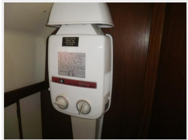
Heater for hot water
