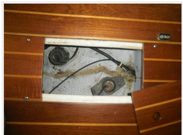
2nd Bilge w/auto Float Switch
