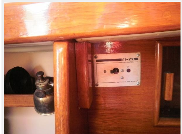
Propane Gas safety Indicator
