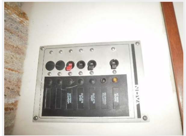
120V House Panel
