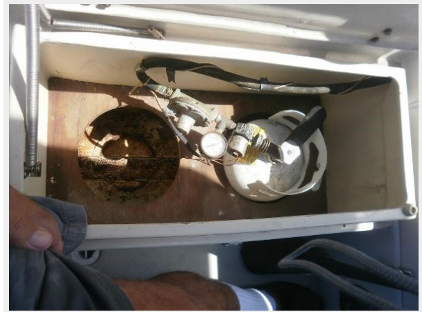
Propane Tank compartment
