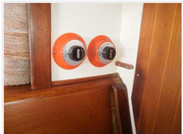
Duel Power Switches w/ Off/ 1/2
