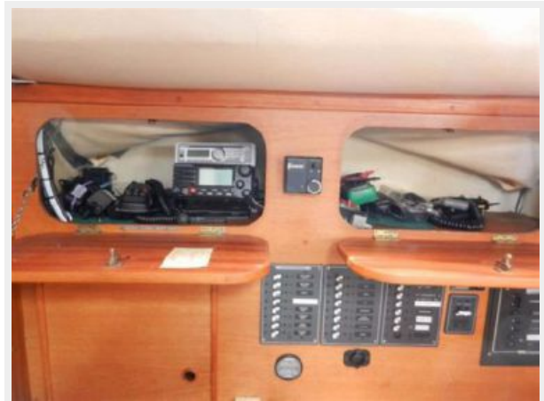
VHF w/AIS and electric panel
