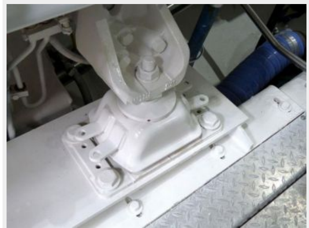
Engine Mount Without Rust
