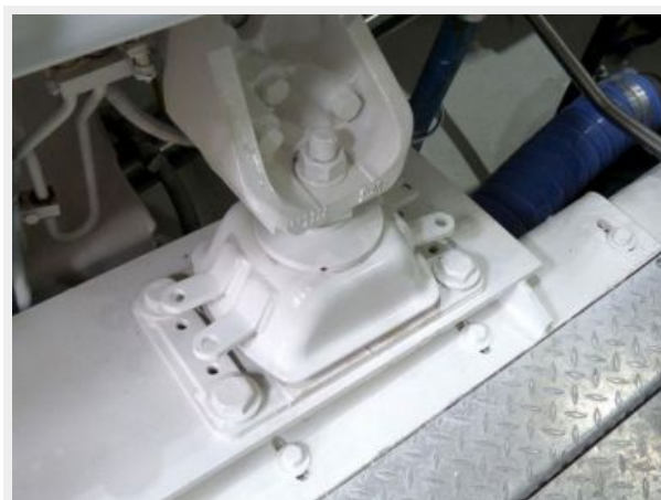
Engine Mount Without Rust
