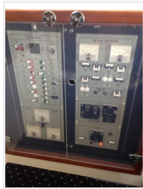
Electrical System / Equipment - Electrical Panel
