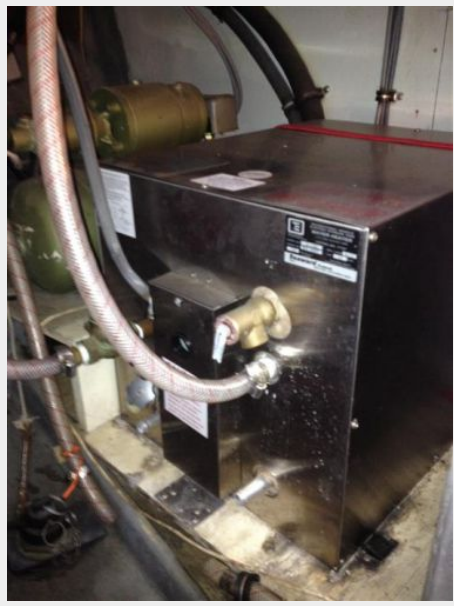
Engine & Mechanical Equipment 3 - Water Heater
