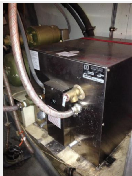
Engine & Mechanical Equipment 3 - Water Heater
