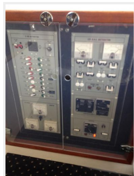
Electrical System / Equipment - Electrical Panel
