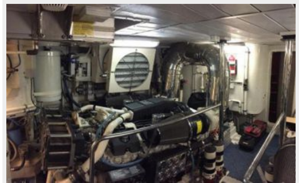
Engine room Pano
