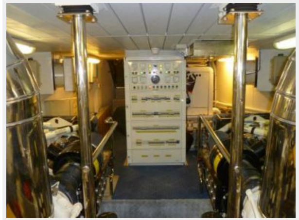
Clean walk in engine room
