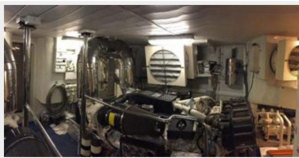
Engine room Pano
