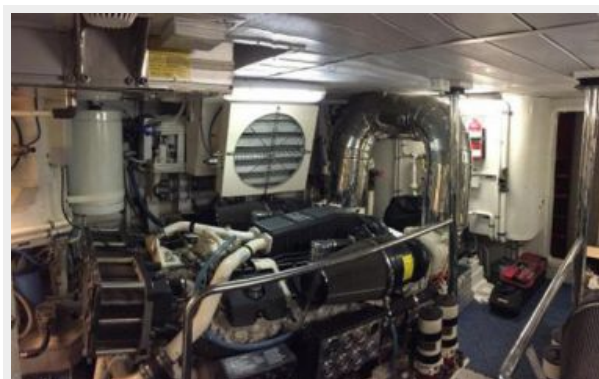
Engine room Pano
