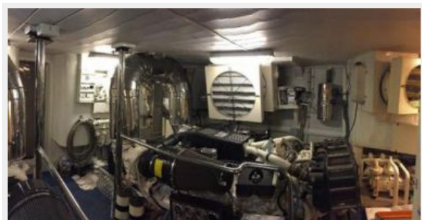
Engine room Pano
