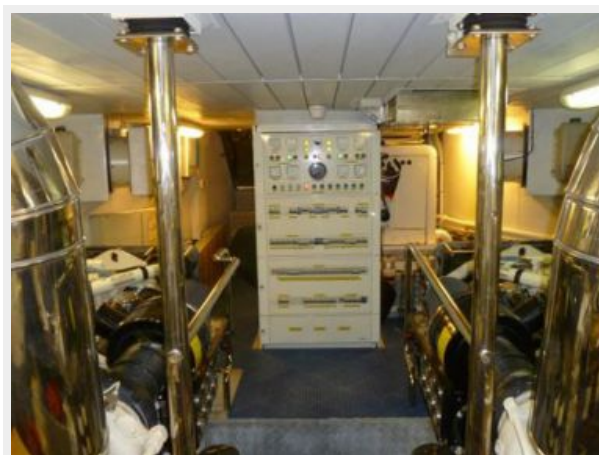
Clean walk in engine room
