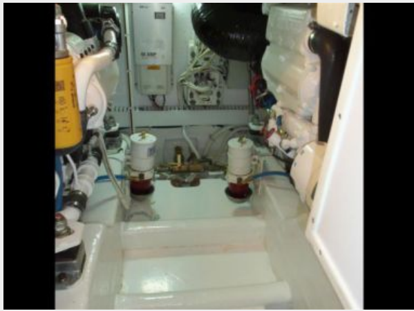
Engine Room Looking Forward
