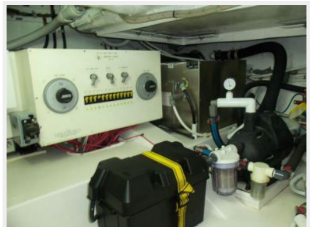
Engine Room Equipment
