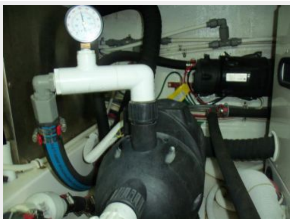
Water Pump & 12 Volt Backup
