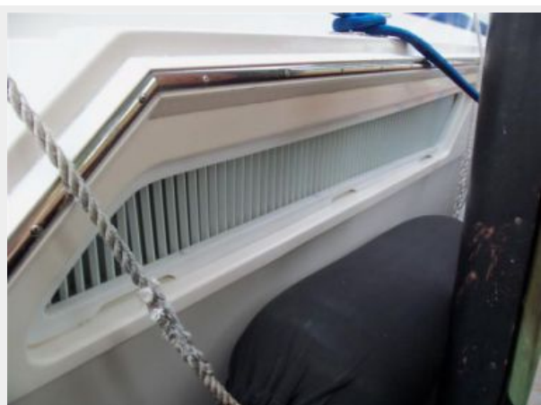
Proper Engine Room Vents
