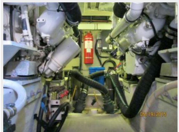
Clean Engine Room II
