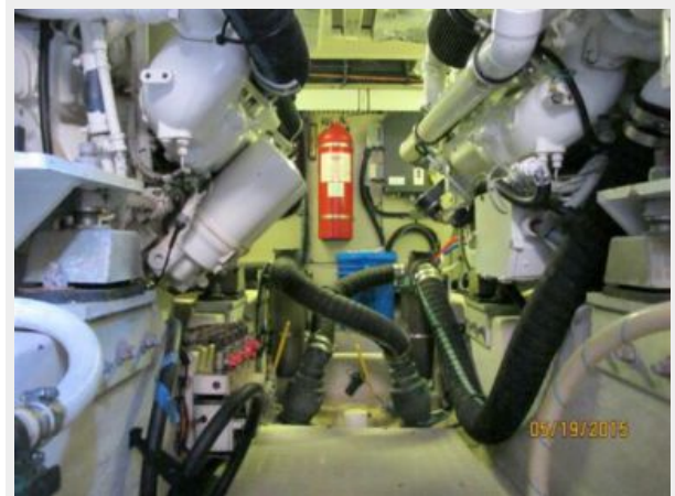
Clean Engine Room II
