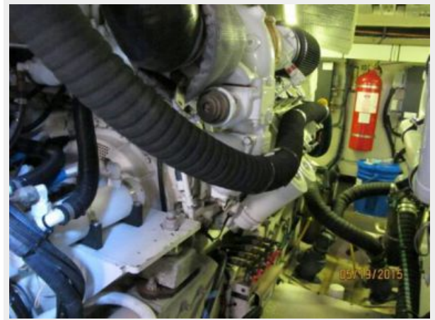
Clean Engine Room III
