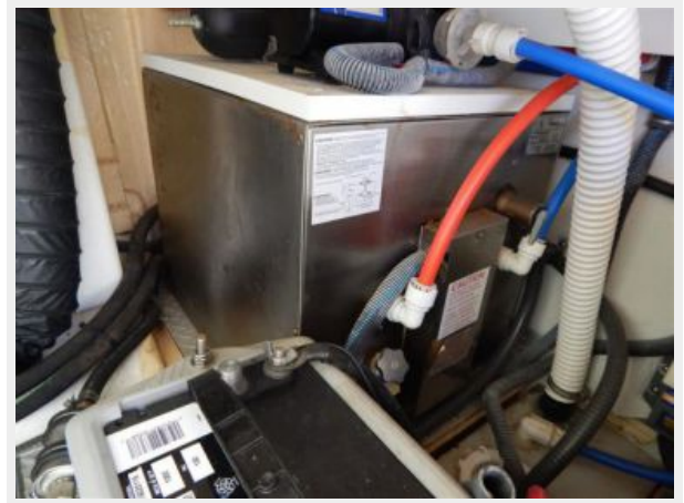
Hot Water Heater
