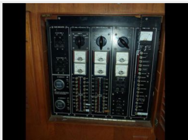
Pilothouse AC Panel
