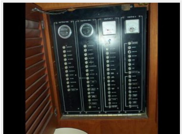
Pilothouse DC Panel
