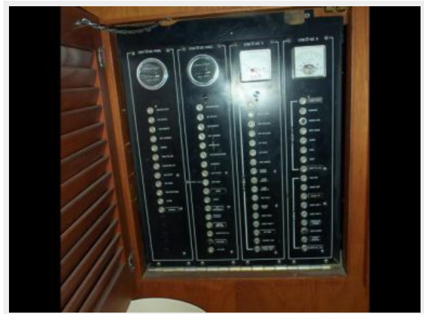
Pilothouse DC Panel
