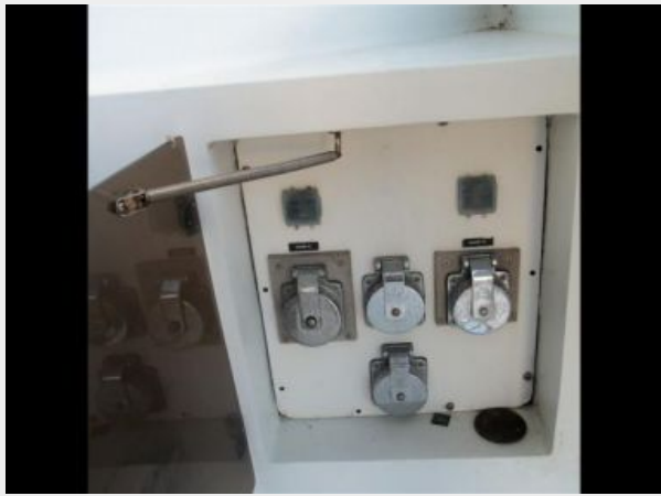
Midship Electrical Service
