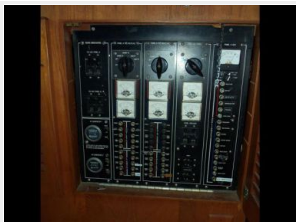
Pilothouse AC Panel
