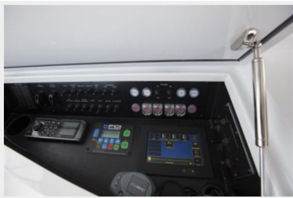
Port Electronics Box
