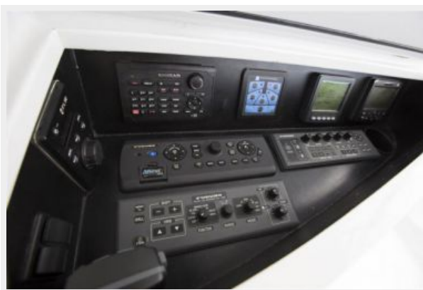
Starboard Electronics Box
