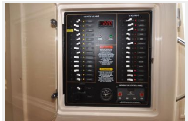
Main Distribution Panel
