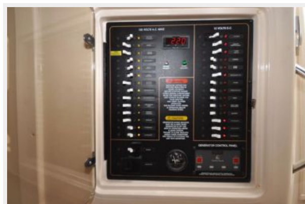
Main Distribution Panel
