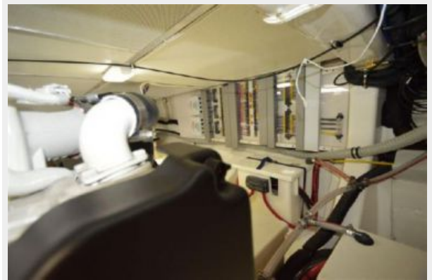
Engine Room Electric
