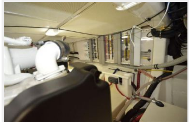
Engine Room Electric
