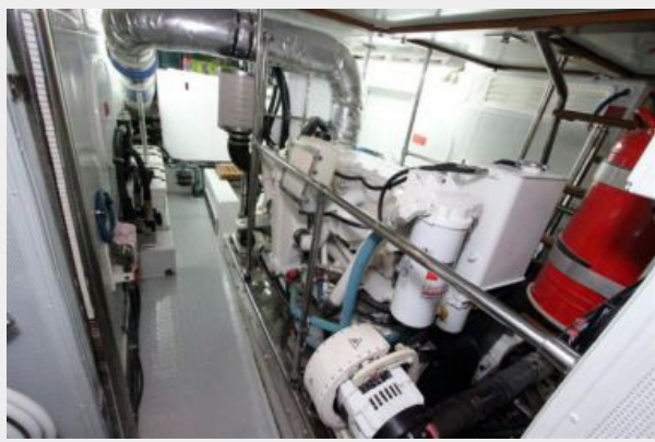
Engine Room Looking Aft
