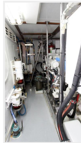
Fuel filtration and Port Engine Room Access
