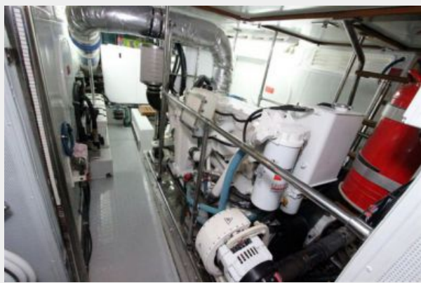
Engine Room Looking Aft
