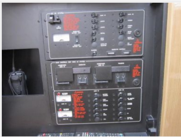
Main Distribution Panel
