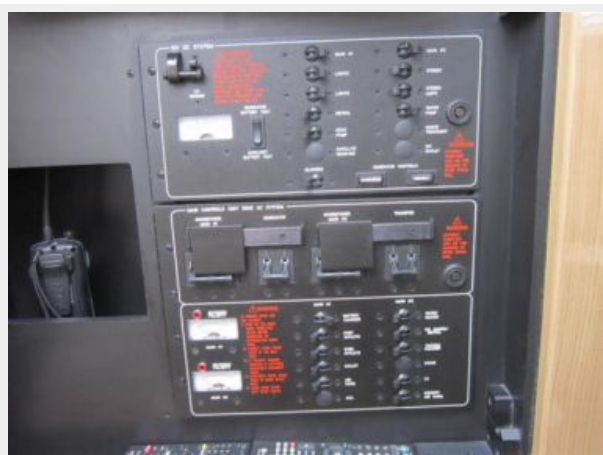
Main Distribution Panel
